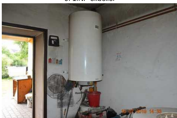
11. 1.NP el. boiler
